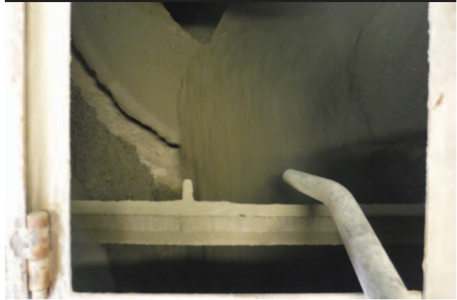
Figure 3: liquid \text{CO}_2 being added to a concrete batch leaving the mixer ( \text{CO}_2 pipe on lower right)
